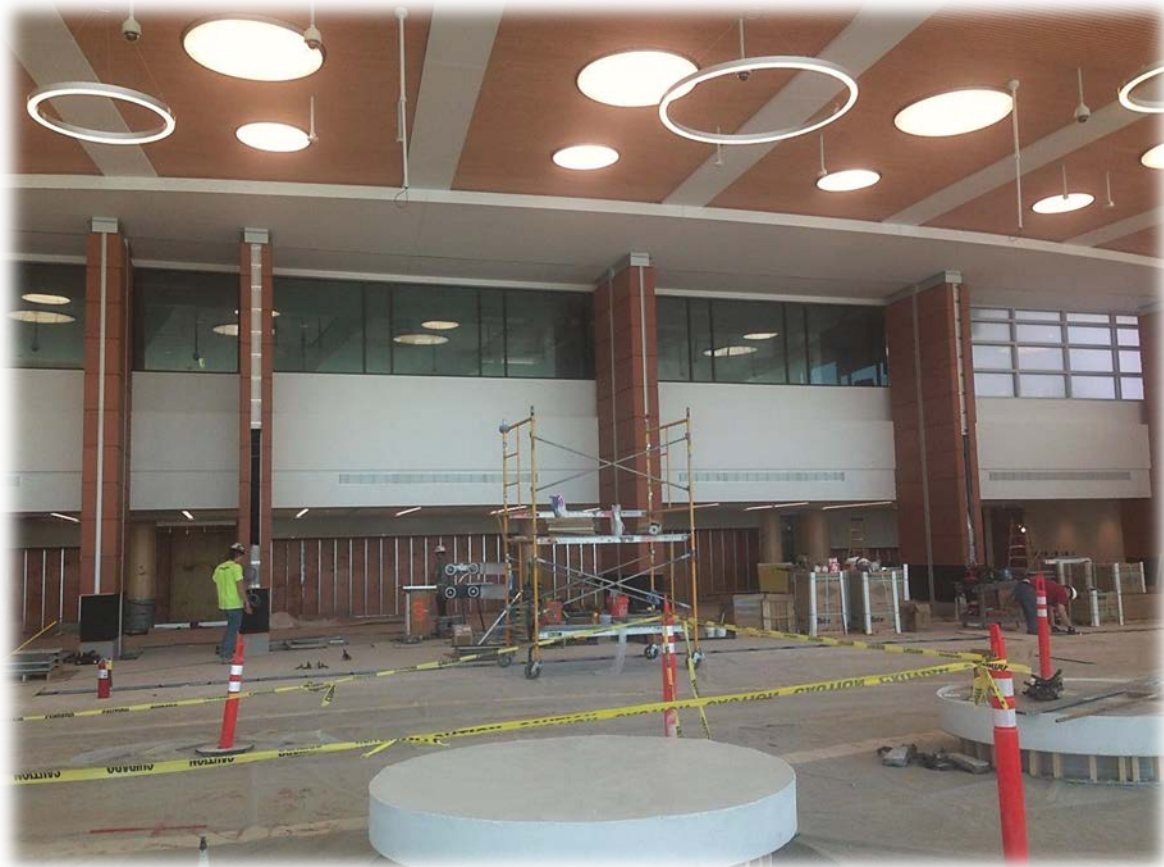
(Above): Construction crews work on the front entrance of the Gateway Transformation Project at the consolidated security checkpoint.
